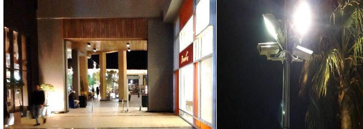
Fig. 4. Security points and CCTV at the parking area.
